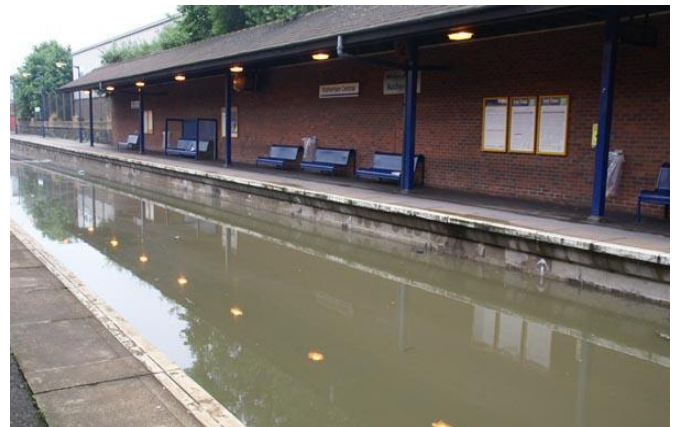
Figure 1. Direct damage in transport sector will imply falls in productivity through commuting delays
